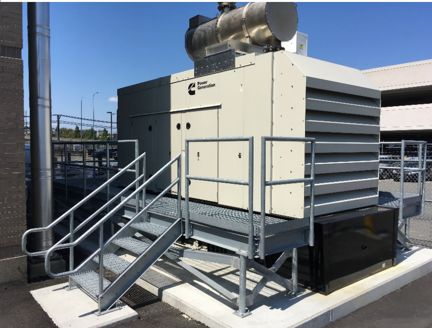
Generator Combo Unit
