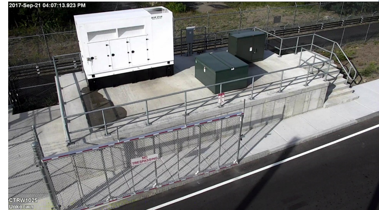
State Police Generator
